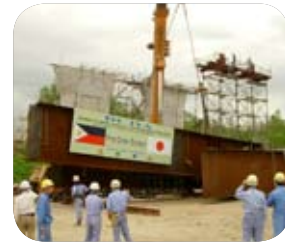
Installation of giant steel girders of the 55-meter high Gumain bridge, the highest bridge of the SCTEx.
